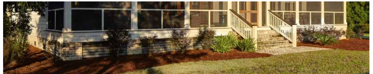
Foundation with louver screening
